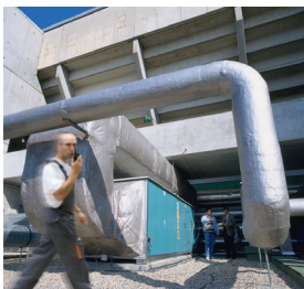
Air handling unit
